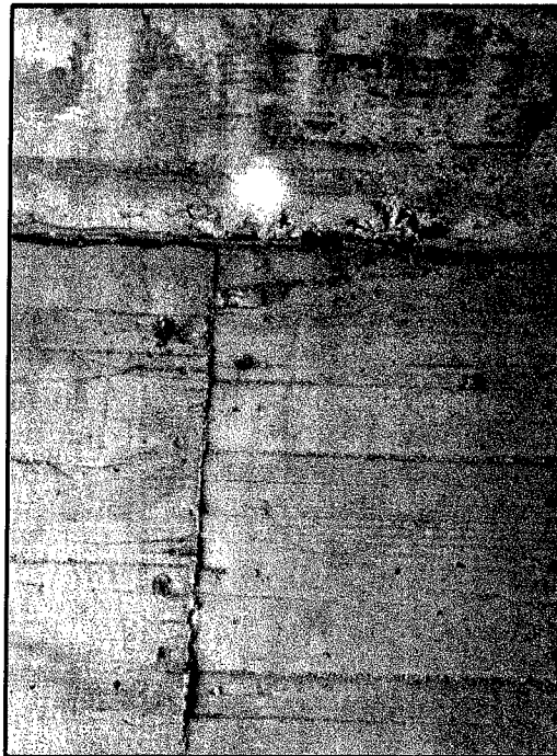
Figure 2. Spalling observed on the bottom of the top slab of the culvert bridge
